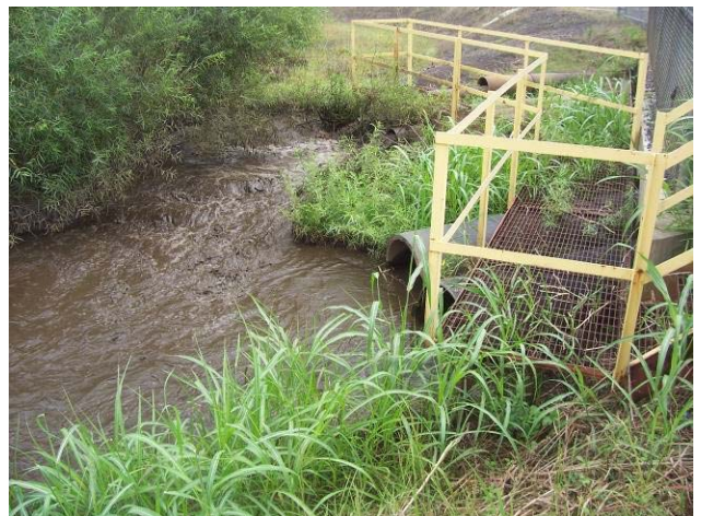
Photo 6 Typical view showing conditions of unobstructed discharge into the fly ash pond.
