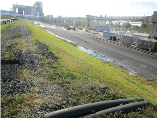
Photo 5 Areas of ponded water along the south dike of the south fly ash pond.
