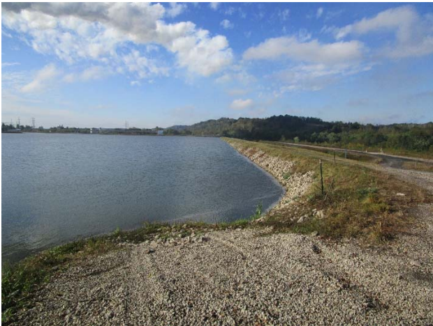
Photo 9 Typical view showing good conditions of the west embankment showing a uniform slope and crest. No erosion of the interior pond slopes was observed.
