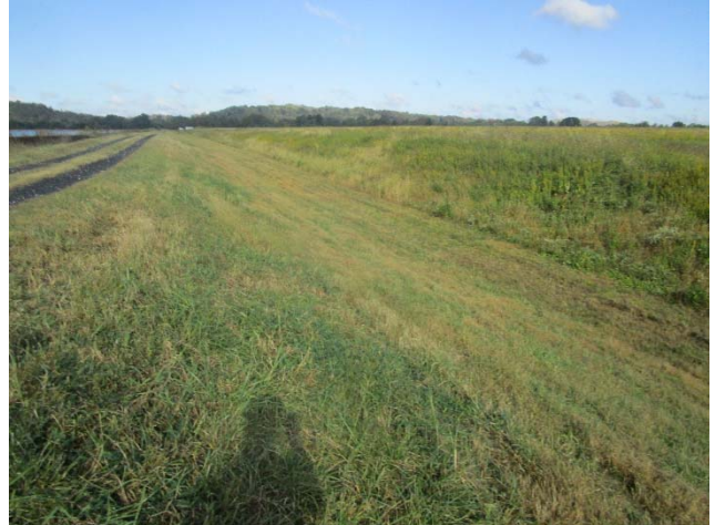
Photo 8 Typical view showing good conditions of the north embankment showing a uniform slope and a well maintained vegetative cover.
