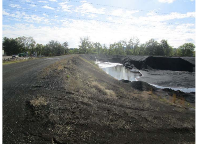
Photo 2 Typical view showing good conditions of the boiler slag embankment and stockpile of material to be used for beneficial utilization.
