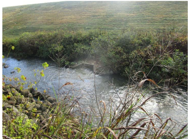
Photo 10 Typical view showing fair conditions of the south fly ash pond discharge structure. Additional mowing is scheduled to be performed within this area.
