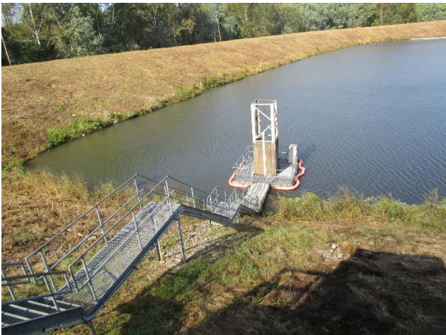
Photo 3 Typical view showing good conditions of the decant structure and interior embankment.
